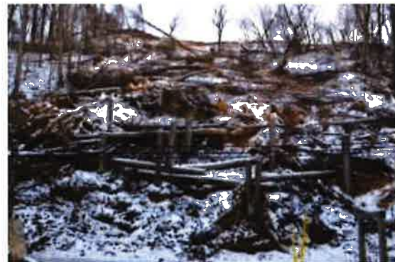
Landslide above Balligomingo Road
